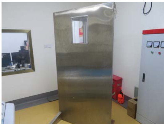
图 3-32 SPECT/CT 机房内铅屏风
